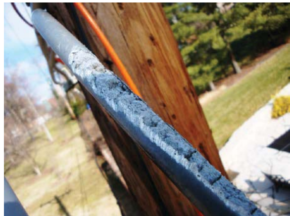
More rodent damage
