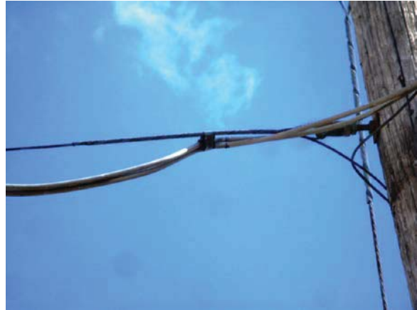
Radial crack in feeder cable
