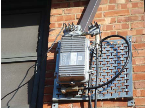
Illegal MDU connection
