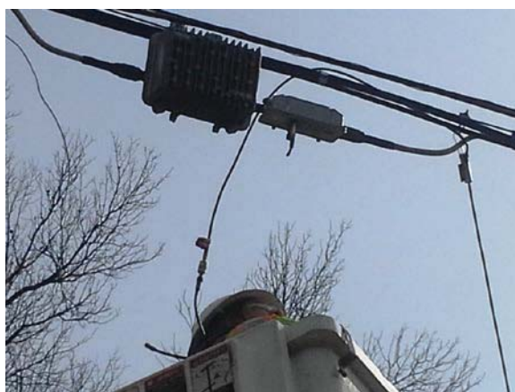
Loose tap faceplate
