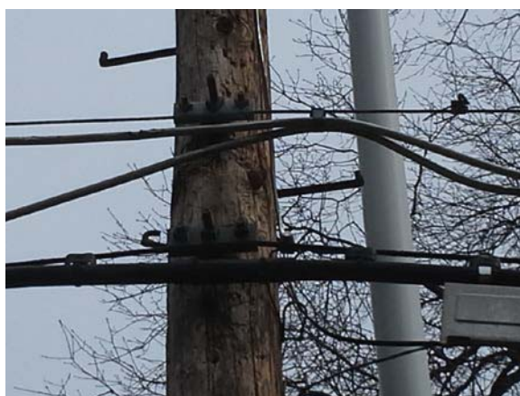
Power line fell on coax, melted shield
