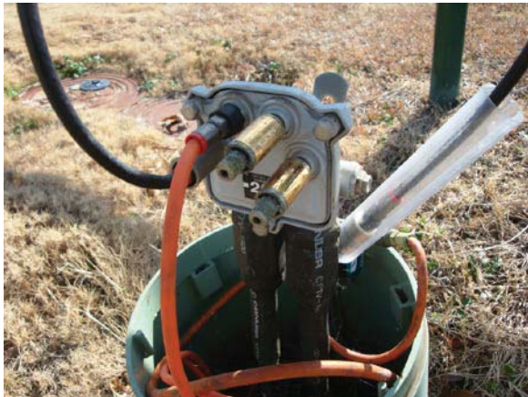
Corroded and loose terminators
