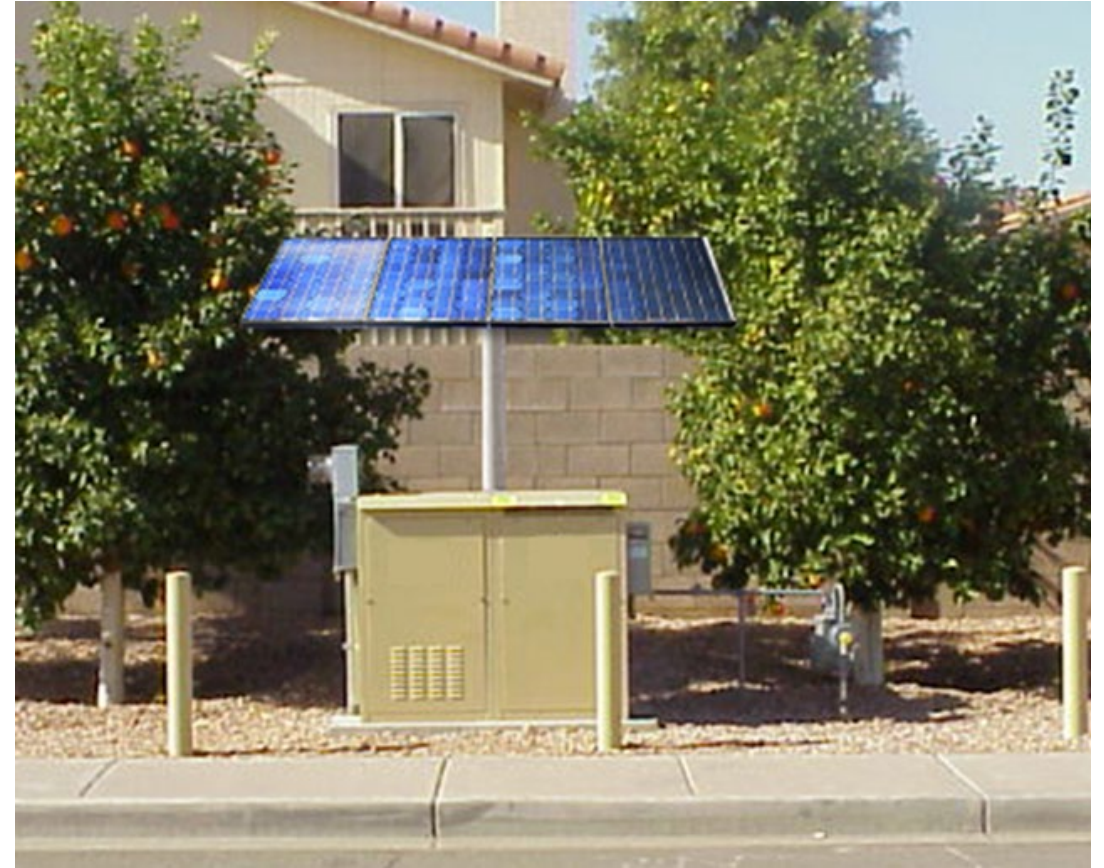
Example of a solar augmented cable power supply
