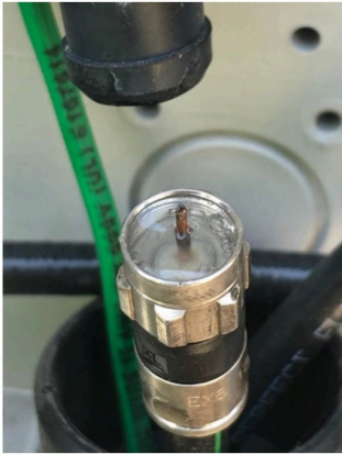
Water coming out of the end of the connector at the ground block
