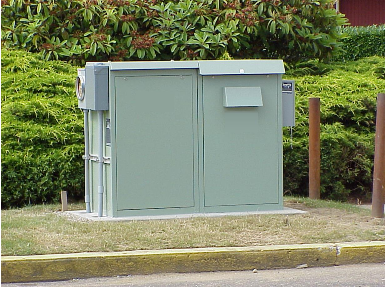
Figure 3 - Typical Curbside Generator Installation Using Natural Gas
