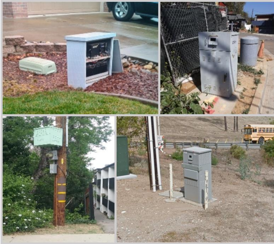
Figure 1 - Example cable broadband powering sites. The variability in available space, loading, and local regulations makes a one-size-fits-all solution for extended run time nearly impossible.
