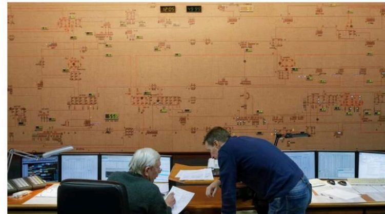
Dispatchers are seen inside the control room of Ukraine's National power company Ukrenergo in Kiev, Ukraine, October 13, 2016. REUTERS/Valentyn Ogirenko
