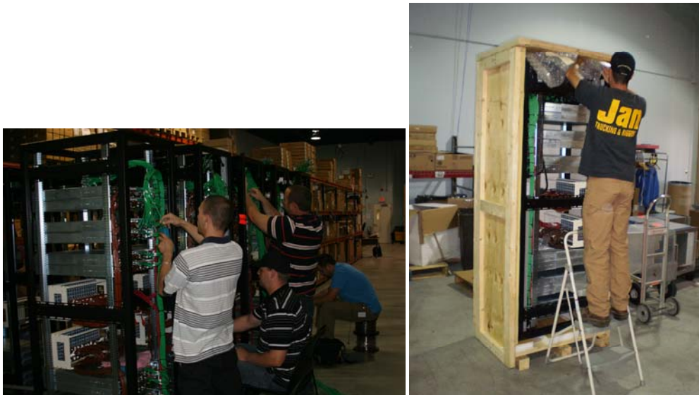
Figure 3: Performing the Rack, Stack, Wiring and Labeling of the SDV Equipment Remotely Offers Advantages Over Onsite Installation
