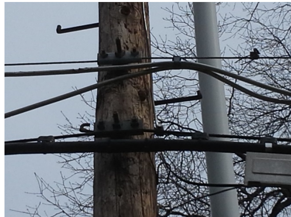
Power line fell on coax, melted shield
