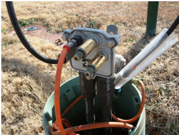
Corroded and loose terminators
