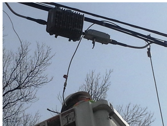
Loose tap faceplate
