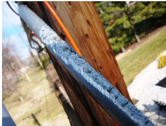
More rodent damage
