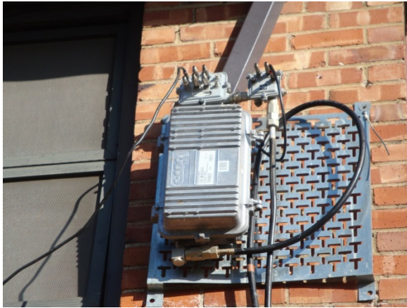
Illegal MDU connection
