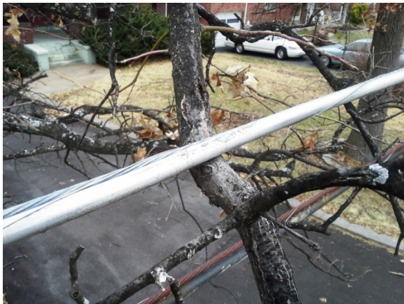
Tree limb rubbing on coax
