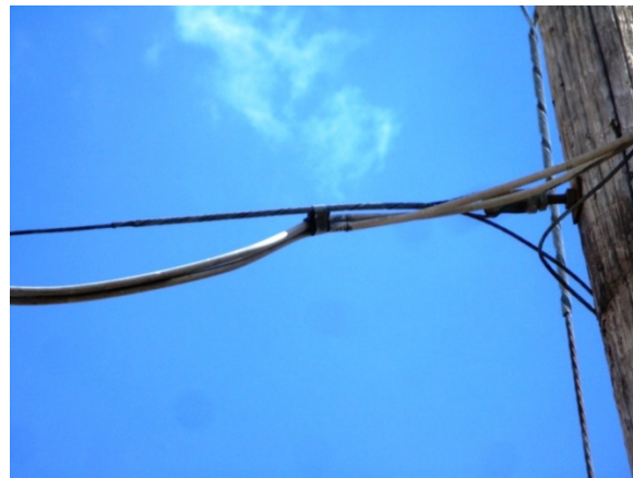
Radial crack in feeder cable
