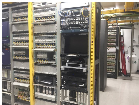
Figure 13 - Site B Server Racks
