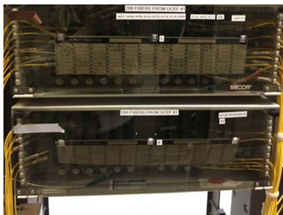
Figure 15 - Site C Server Racks
