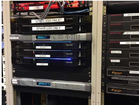
Figure 11 - Site A Server Racks
